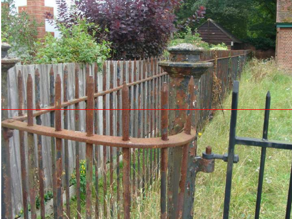
Picture 16 — Metal fence to side of Thames Water facility, worthy of retention and in need of repainting.
