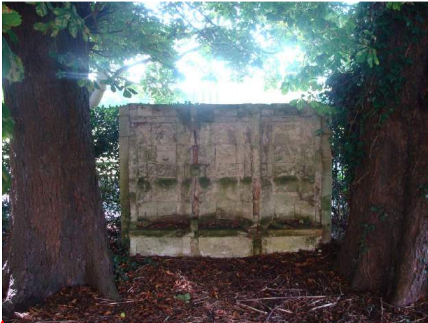
Picture 43 – 14 th century grade II Sedilia removed from church during 19 th century 'restoration', now in need of urgent repairs. Included on the Council's BuildingsHeritage at Risk Register.
